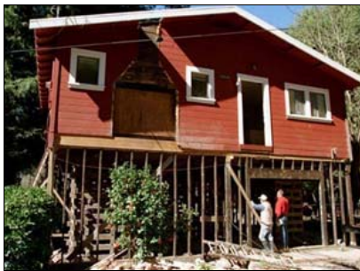
Guerneville, CA, April 23, 1998 -- Mitigated (elevated) home along the Russian River. FEMA News Photo
